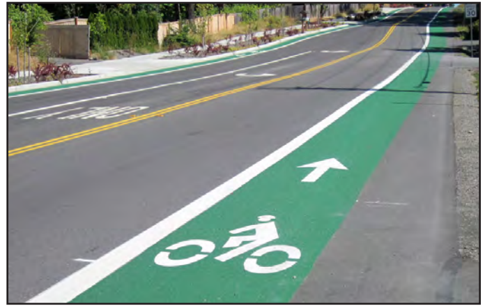
An example of a "greenlane" striping that can be added for a bicycle lane
